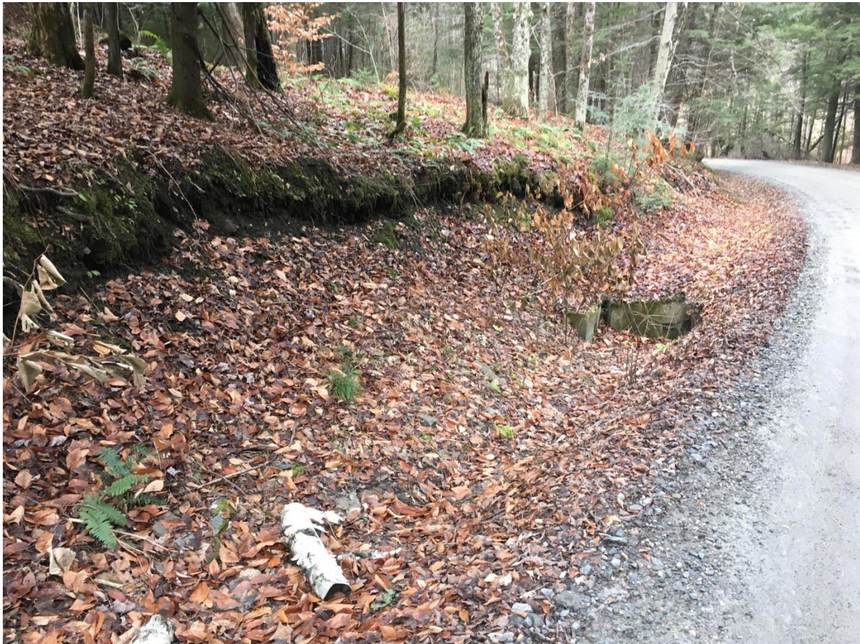
Erosion at inlet
