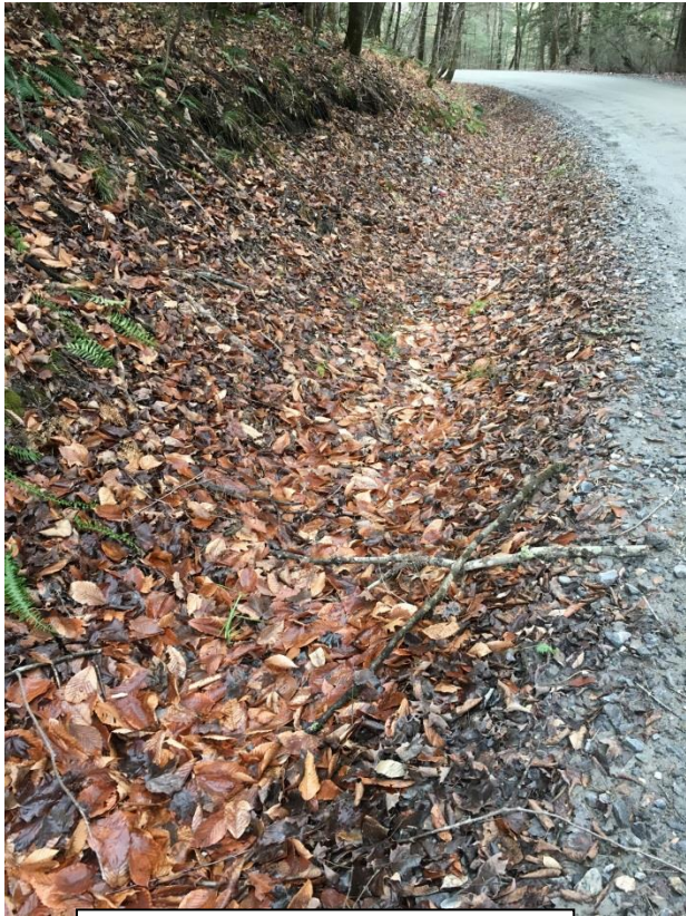
Erosion downhill of culvert inlet
