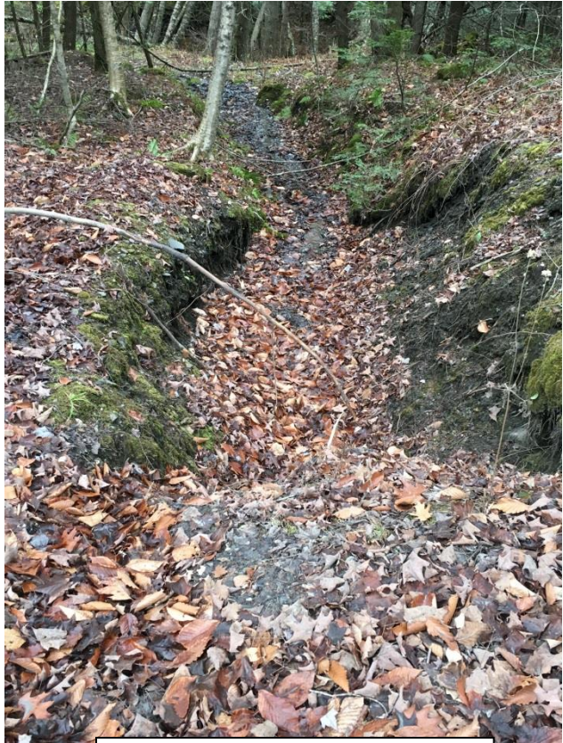
Erosion at culvert outlet
