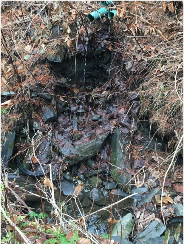
Small drainage sources causing erosion
