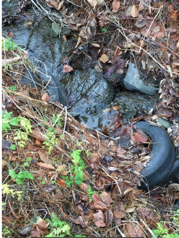
Tires in Inlet Ditch
