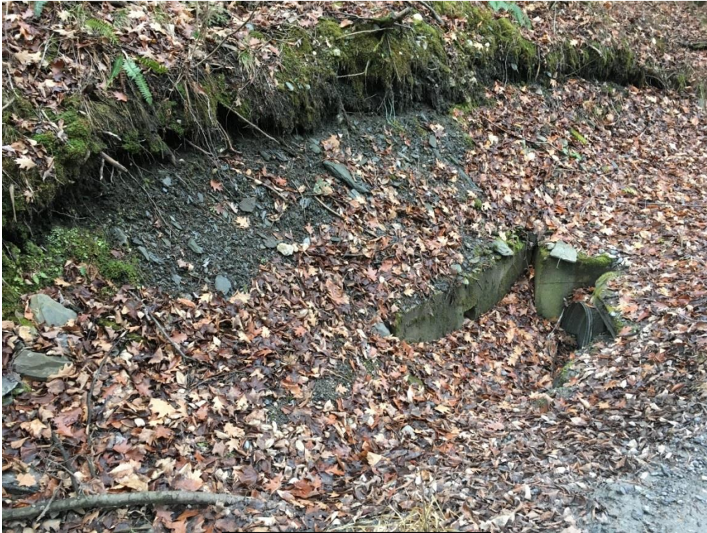
Erosion at culvert inlet
