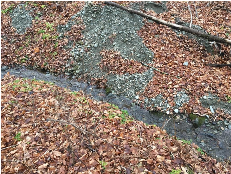
Peth Road: Sediment Buildup at Inlet
