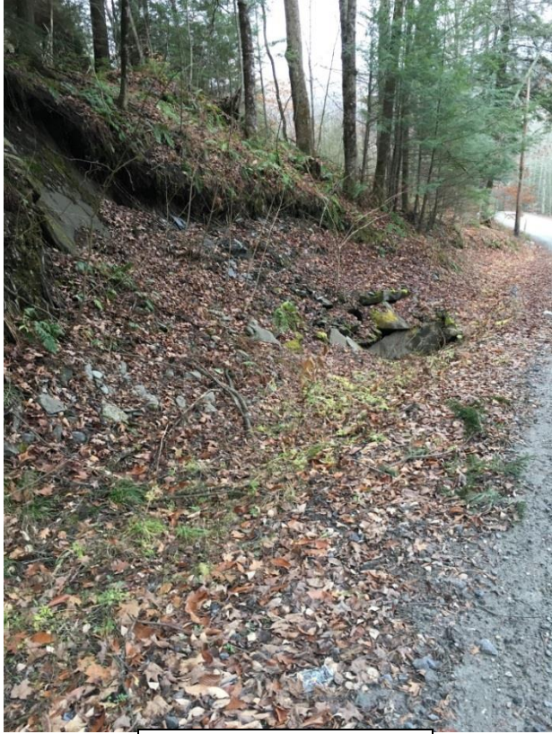
Erosion at culvert inlet
