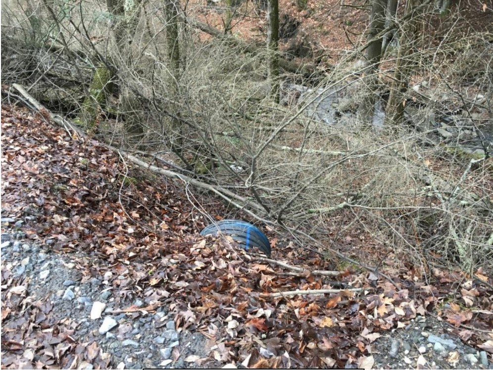
Outlet discharge to surface waters
