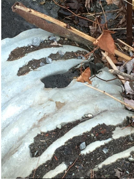
Broken Part of Outlet
