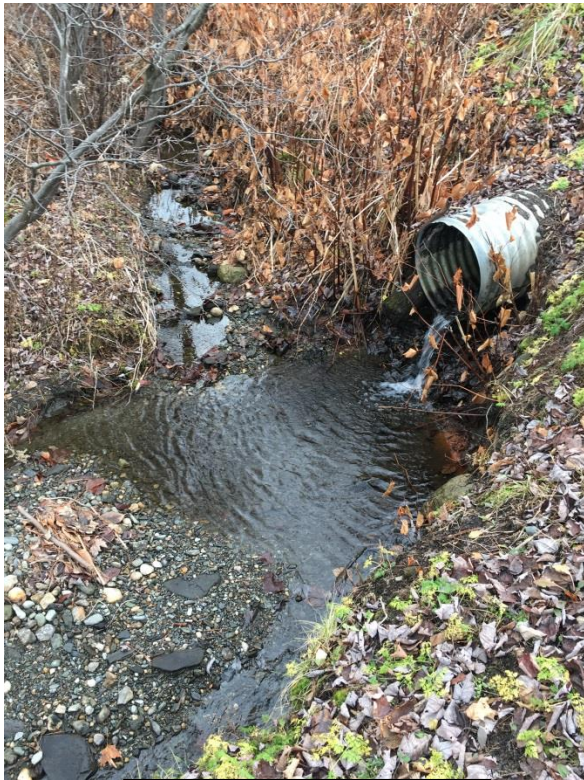
Perched Culvert Outlet
