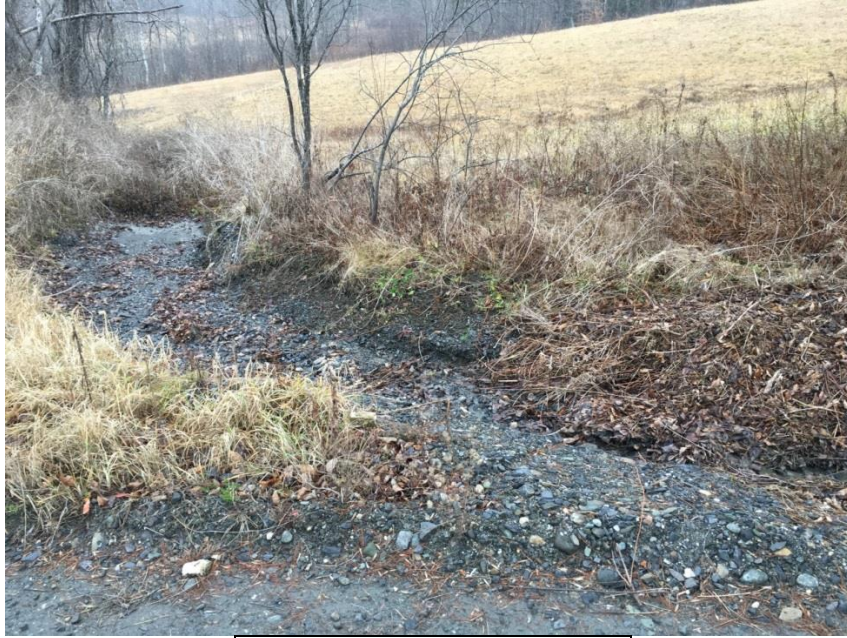
Road Washout from Stormwater Runoff
